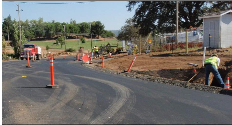
McCourtney Road at Adair where the project improves sight distance and straightens the curve
