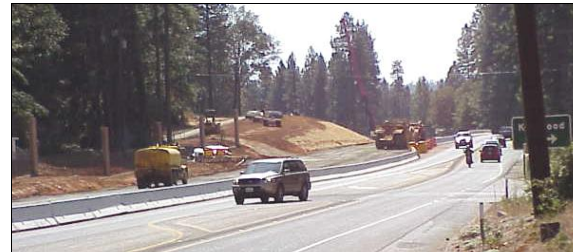
SR 49 widening near Kenwood Ave. with soundwall posts in place and adjacent ground being readied for asphalt
