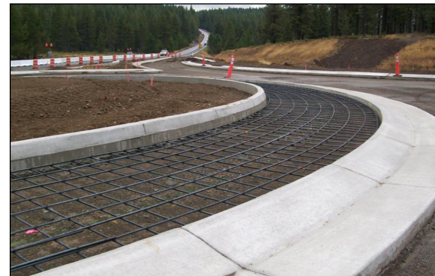
Alder Drive Roundabout underway at the intersection of SR 89 N and Prosser Dam Road
