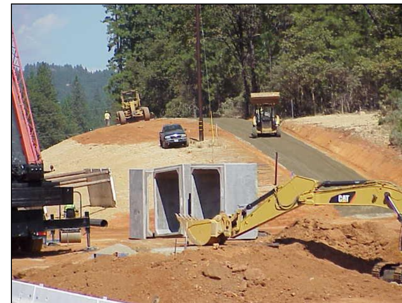
The contractor prepares to install concrete boxes for a deer crossing on SR 49
